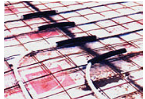
Radiant concrete slabs should be well insulated. Tubing is tied to reinforcing wire mesh and is protected by PVC sleeves where it passes beneath walls and control joints.
