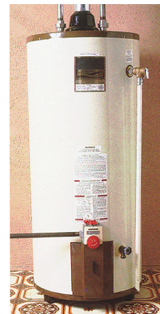
Water heaters can accumulate rust and sludge. Iron and sulfur bacteria can create sulfur odors in water heaters.
