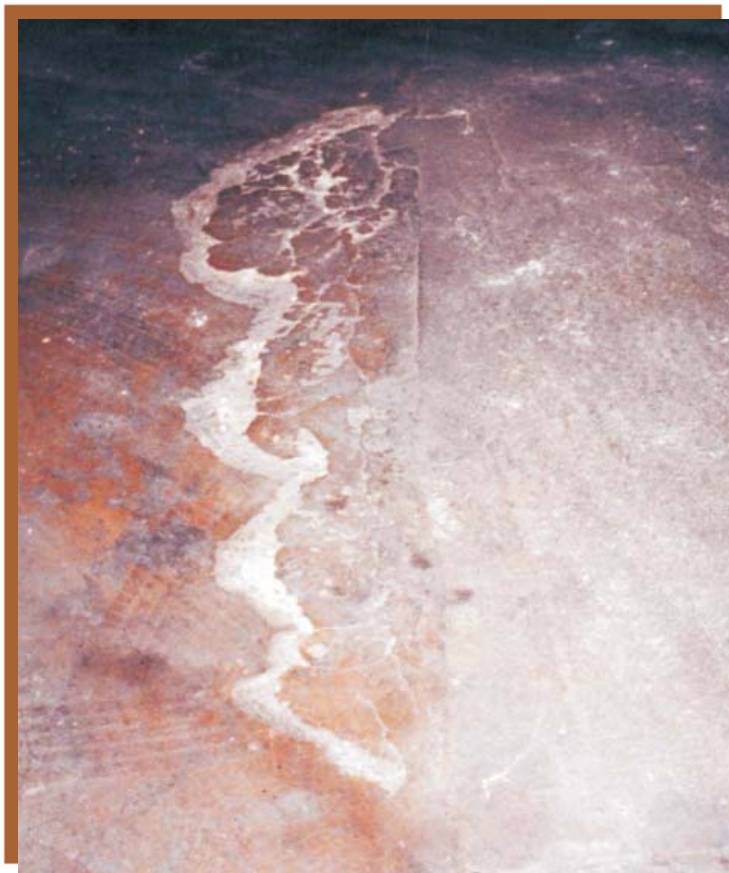
The Guide has been updated to include new technology. For example, delamination of concrete around the perimeter of repair patches due to the “halo effect”, as shown above, is a common problem that can occur within years after the repairs are completed. New strategies to delay the onset of the “halo effect” have been added to the Guide.
