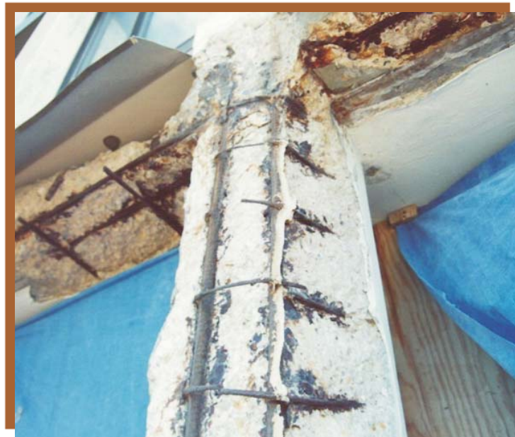
The Guide provides assistance for repairing deteriorated columns as shown above, as well as for other concrete elements
