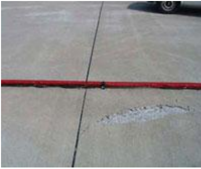
Buckling occurred at Fort Campbell after one slab compressed against another. Photo courtesy of ERDC-CERL.
