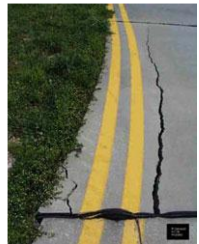
One slab tore another after the cumulative effects of alkali silica reaction at Fort Campbell, Kentucky. Photo courtesy of ERDC-CERL.
