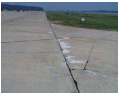
Pictured is an overview of alkali silica reaction damage common to colliding slabs, which took place at Fort Campbell, Kentucky Army Airfield. Photo courtesy of the Army's Engineer Research and Development Center (ERDC) Construction Engineering Research Laboratory (CERL).
