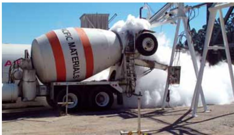
(below) Liquid nitrogen cooling is sometimes used to reduce the temperature of the concrete prior to the time of placement.
