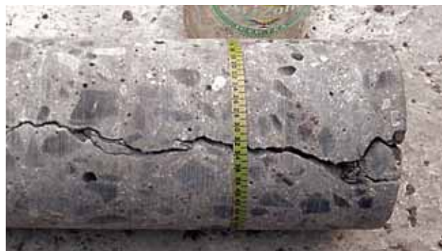
A concrete core removed from a column foundation shows the extent of thermal cracking.
