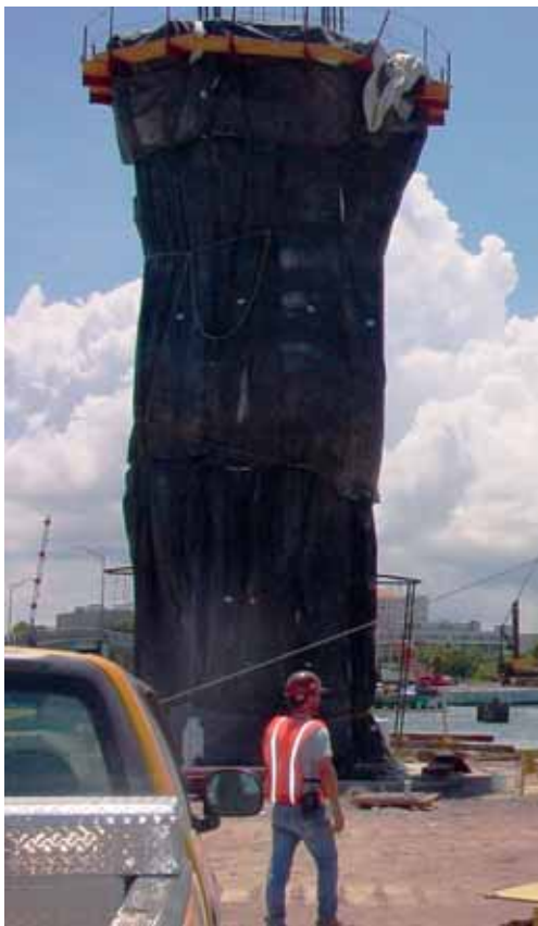
(left) A bridge column uses surface insulation to minimize the temperature difference between the interior and the surface.
