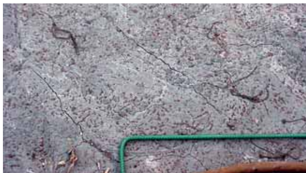
Example of severe thermal cracking on the top surface of a column foundation.
